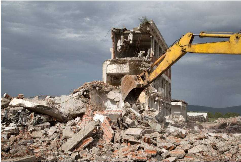
Figure 6. Demolitions of a building. The concrete is grinded down into smaller pieces, during which process some of the paint may form microplastics or particles that spread to the surrounding environment.
